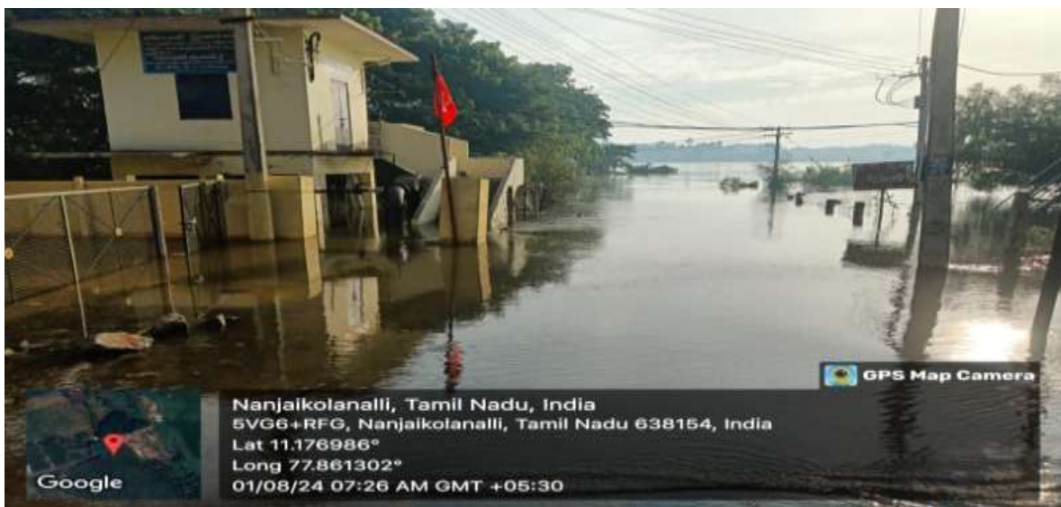
CWSS to Modakurichi Old- Infiltration well submerged
